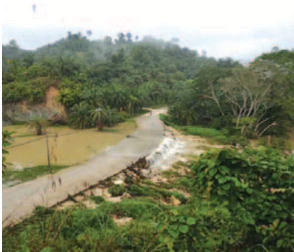
Condition of the Road at Kampung Upak, Lahad Datu, Sabah and cement crossing
